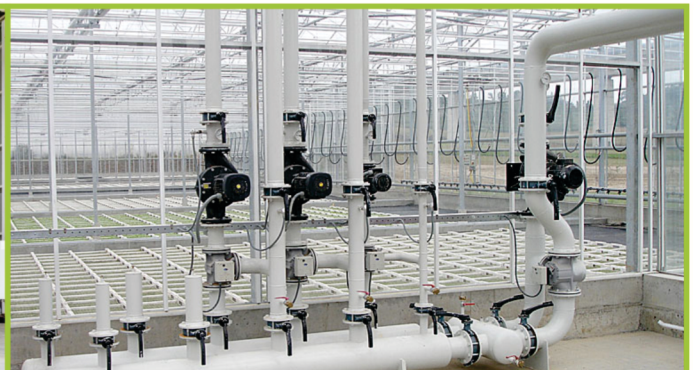
Radiant Heating System
