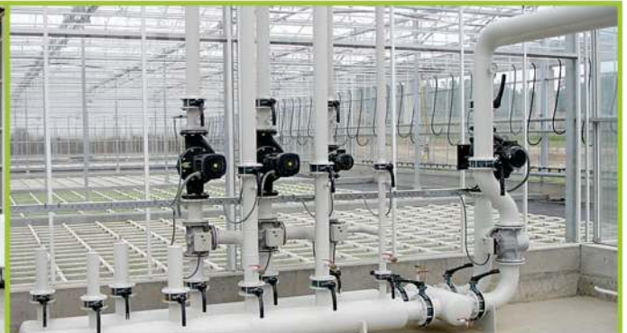
Radiant Heating System
