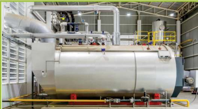
Boiler Heating System
